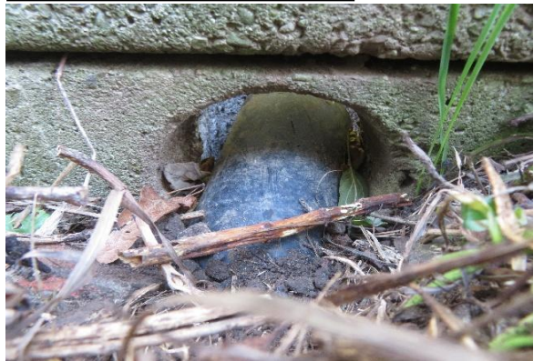
Exposed drain and waste line
