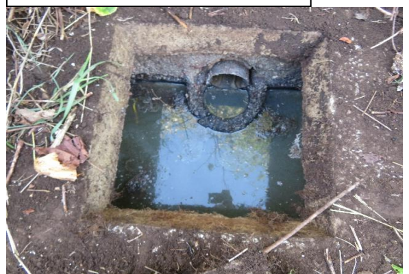
No effluent filter at outlet
