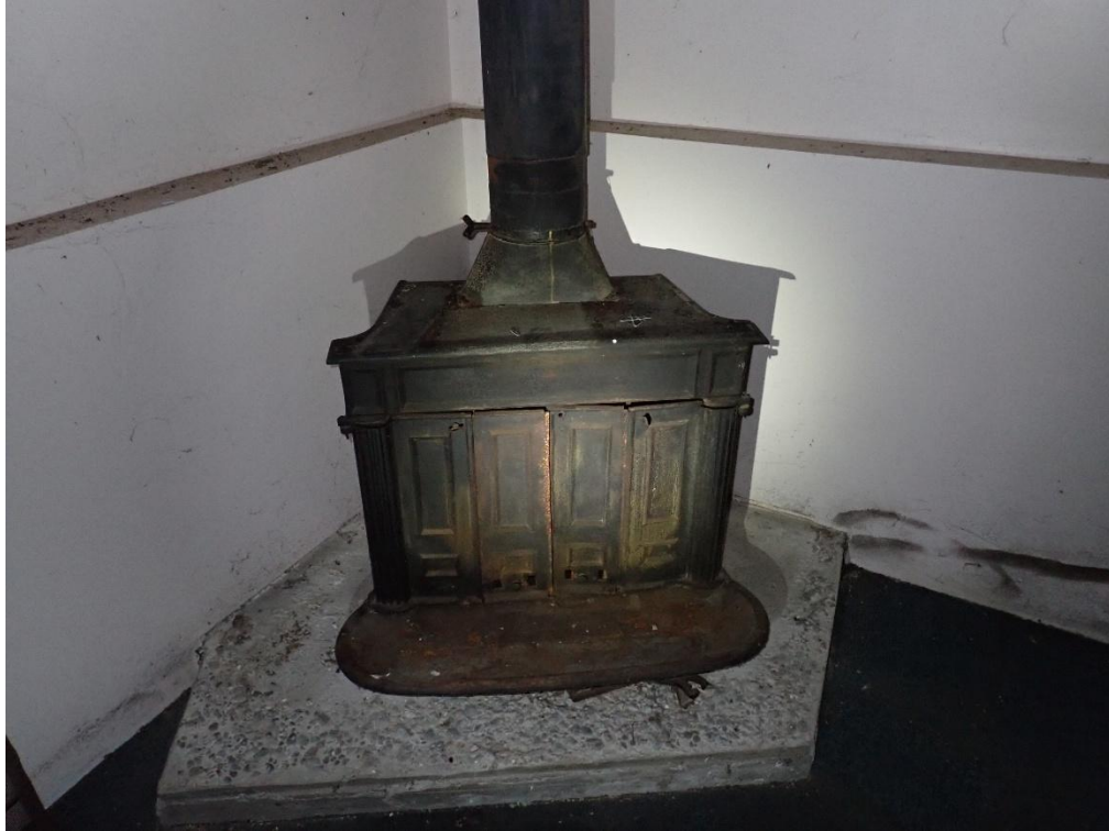
526 Sanford St – Basement Woodstove Overview
