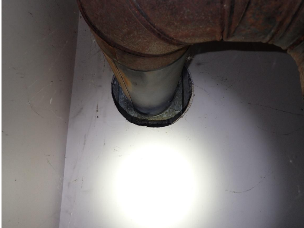
526 Sanford St – Inadequate Clearance Between Flue Pipe and Combustible Materials
