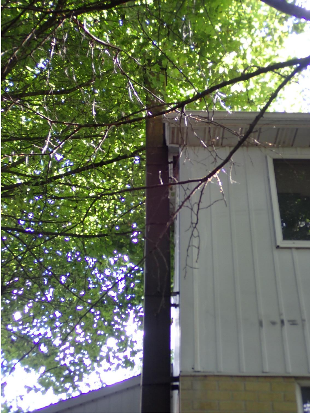
526 Sanford St – Leaning Chimney Sections
