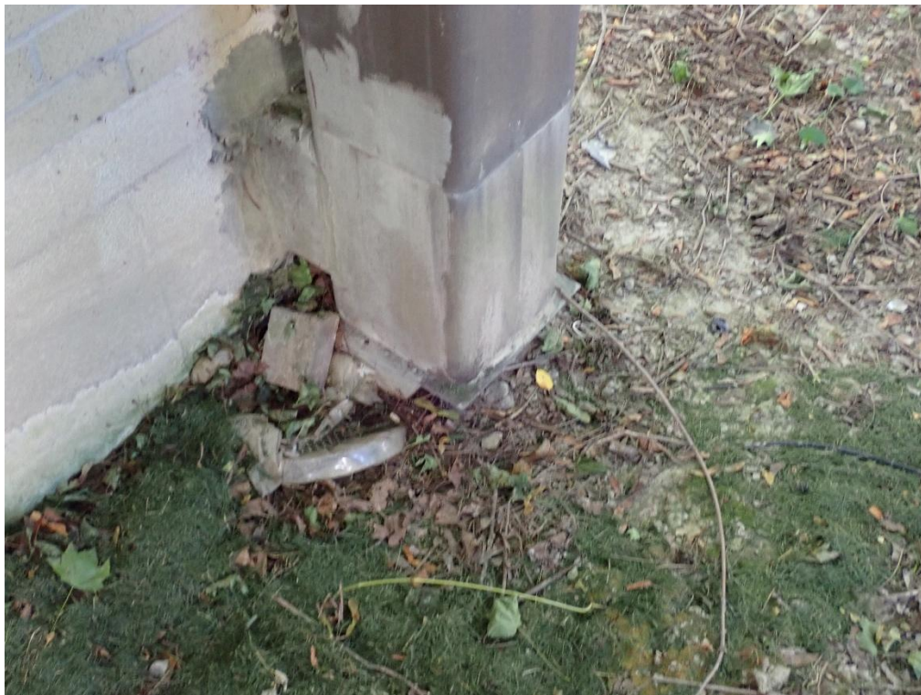
526 Sanford St – Inadequate Clearance Between Base Tee and Grade
