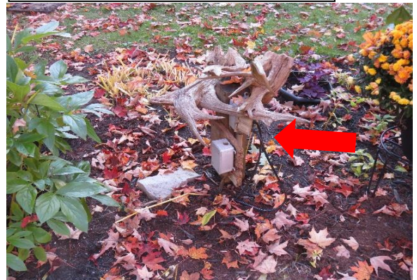
Electrical outlet at pump chamber
