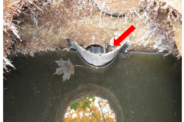
No effluent filter at outlet
