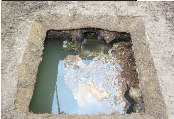
No effluent filter at outlet
