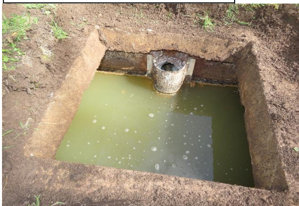
No effluent filter at outlet
