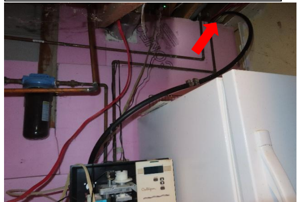
Water filter discharge
