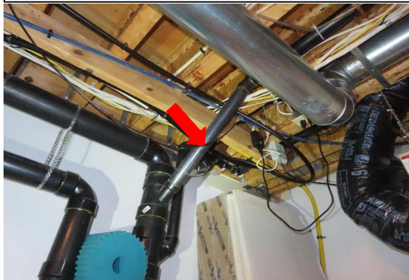
Water filter discharge to septic
