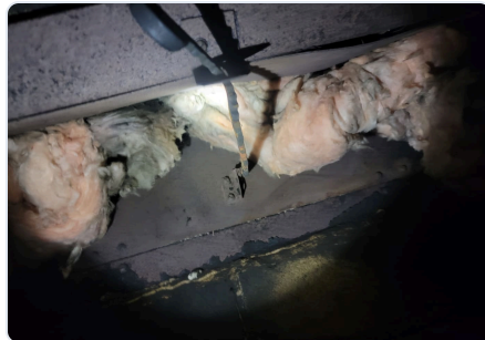
Basement fireplace smoke chamber — fibreglass insulation stuffed into throat/hatch opening
