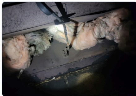
Basement smoke chamber/throat — fibreglass insulation packed into opening, damper obscured
