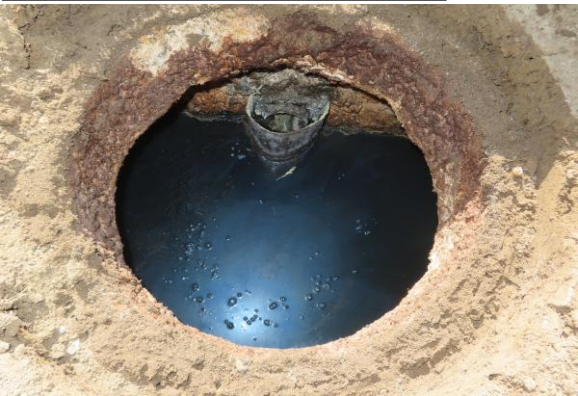
No effluent filter at outlet
