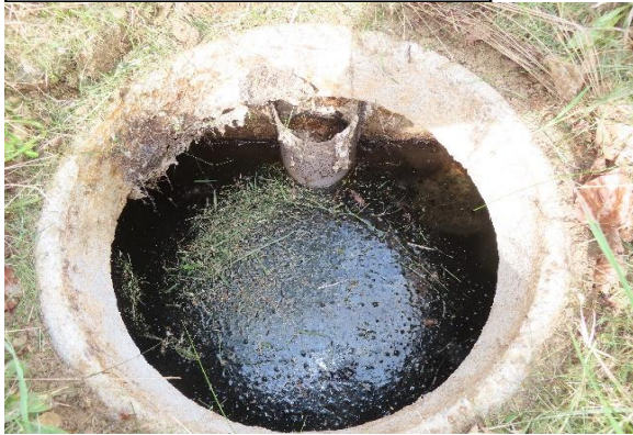
No effluent filter at outlet
