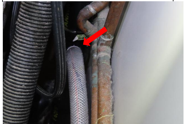
Water filter discharge to septic
